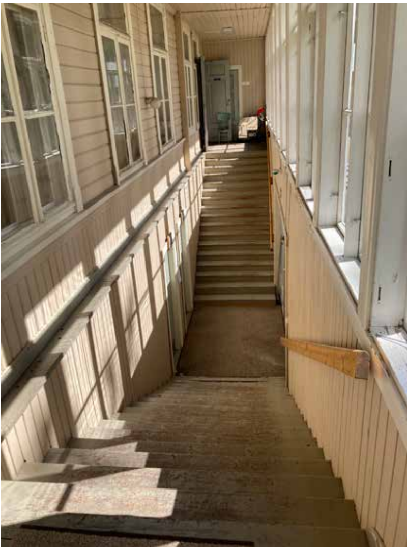
The porches in the courtyard entrance were connected when the toilets were installed in the basement.
