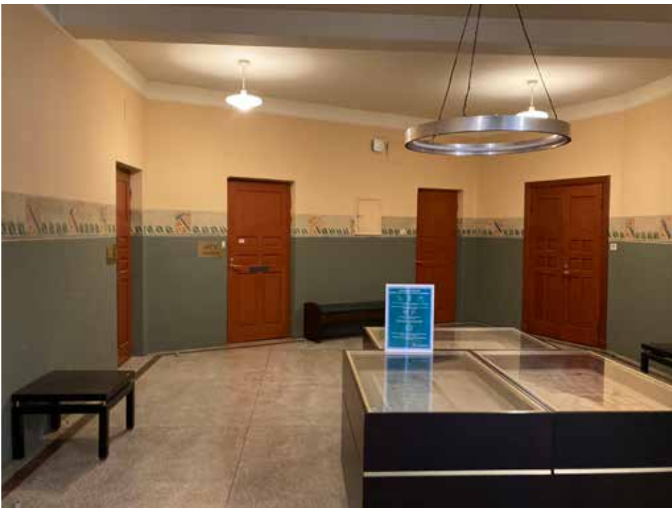
The lobby of the office floor. New lamps beside the old ones bring extra light to the lobby.
